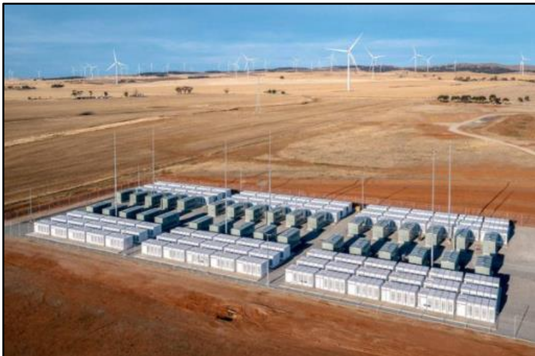
Figure 3 – Wind turbines and battery facility at Hornsdale (image courtesy of the Applicant)
